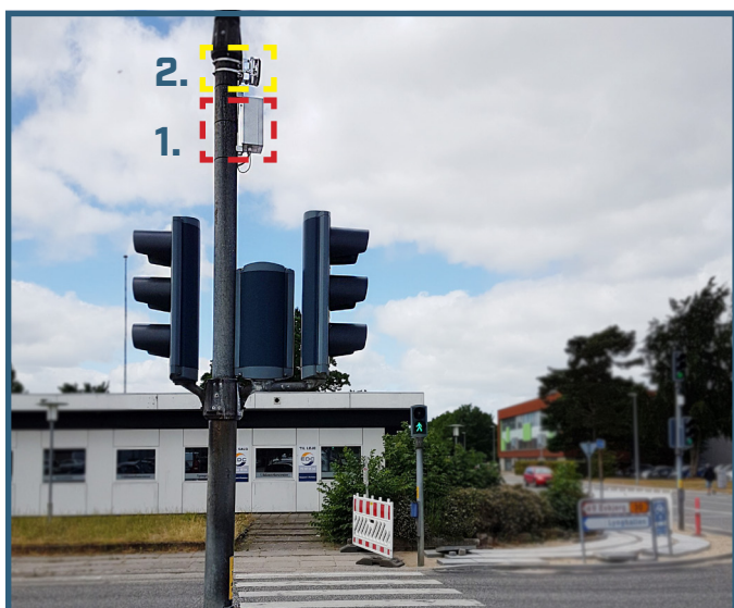
The Anybus Wireless Bridge II (1.) is connected to the radar (2.) via a single serial cable and paired with another Anybus Wireless Bridge II in the control cabinet.
