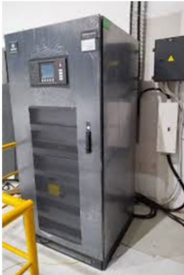
Vertiv's legacy UPS system
