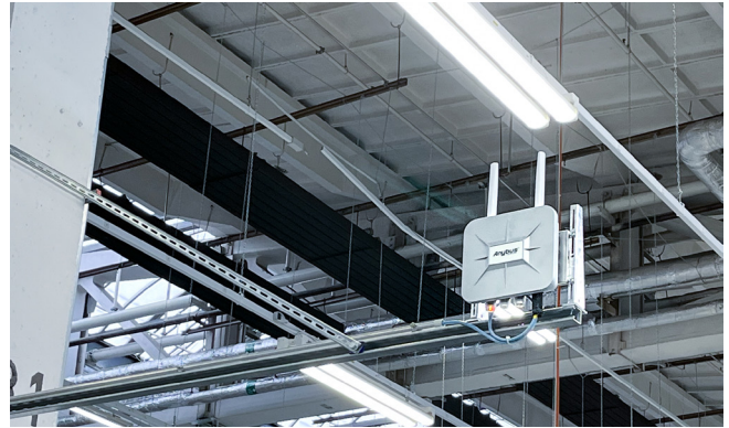
Access Points were strategically placed around the factory to ensure seamless connectivity.
